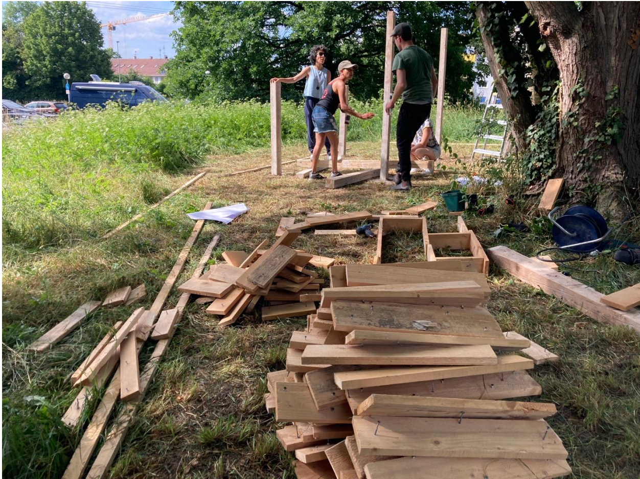
Figure 50 Using the crowdsourced wood materials to create the main structures of the greenhouse. Photo by Anna Szilágyi-Nagy.
