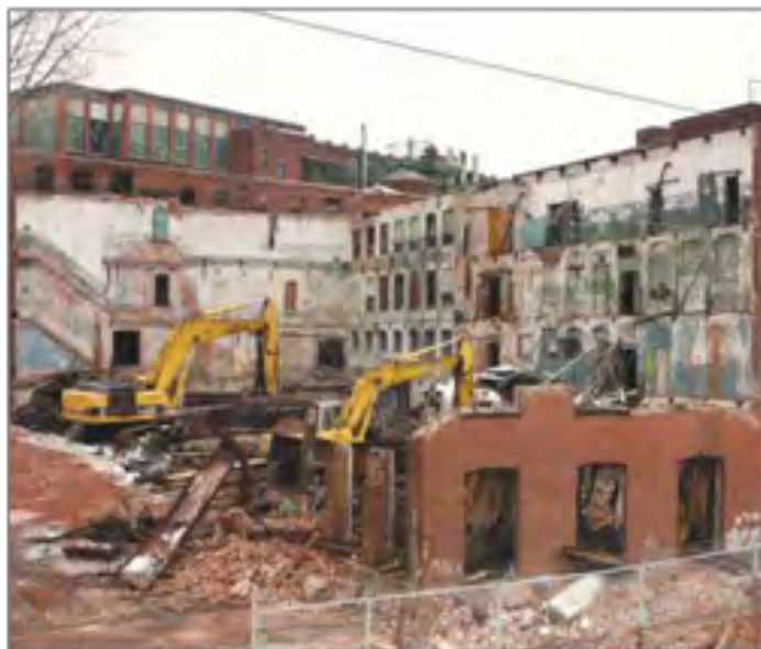
A scene from the recent demolition of six buildings at the Uniroyal/Facemate property site.
